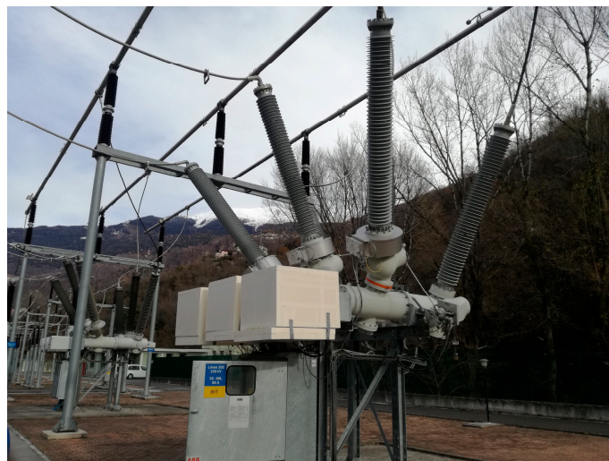
Figure 17. TSG with drives shielded by polystyrene enclosures.
